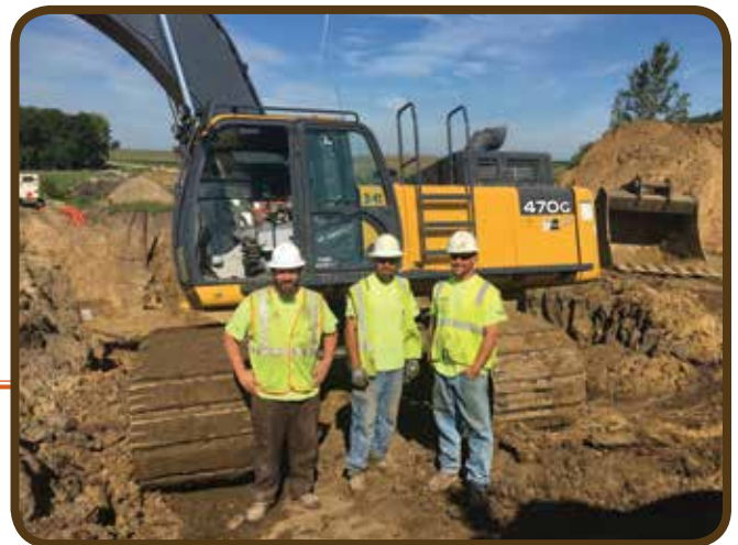
Brothers Lincoln Taylor, Seth Skelton and Curtis Petersmith doing some pipework on the Highway 120 project for Dave Schmitt Construction
