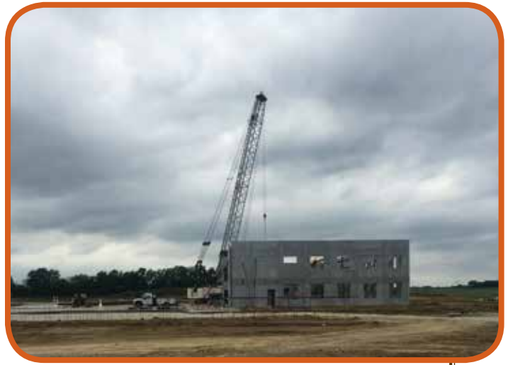
Northwest Erection setting precast at Baker Electric's new office/shop in Des Moines
