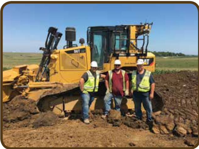
Brothers Chad Tesar, Chisolm Laird and Jessi Alexander working on the civil portion of the Ida Company Wind project for Mortenson
