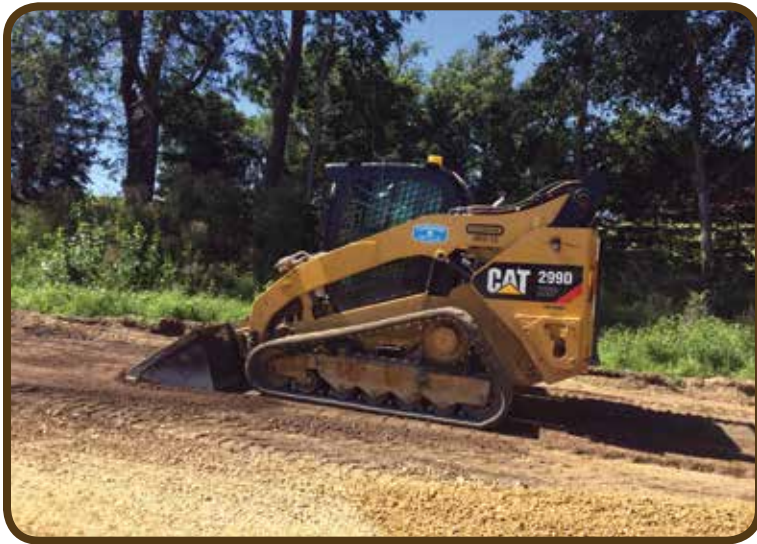
Apprentice Sam David operates a Cat 299 Skid Loader for Tschiggfrie on a road project north of Dubuque
