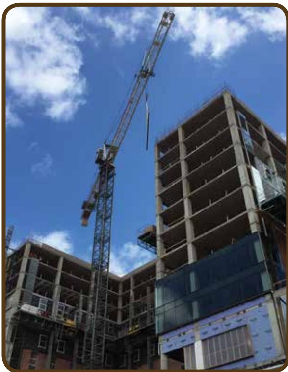
Brother Ben Bunn operates a tower crane at the University of Iowa dorm project in Iowa City for Miron. Brother Shawn Wilson (not pictured) operates the second tower crane on this project
