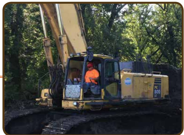
Brother Larry Buck operates a Komatsu PC 800 Excavator for SM Hentges at a sewer project in Cedar Rapids
