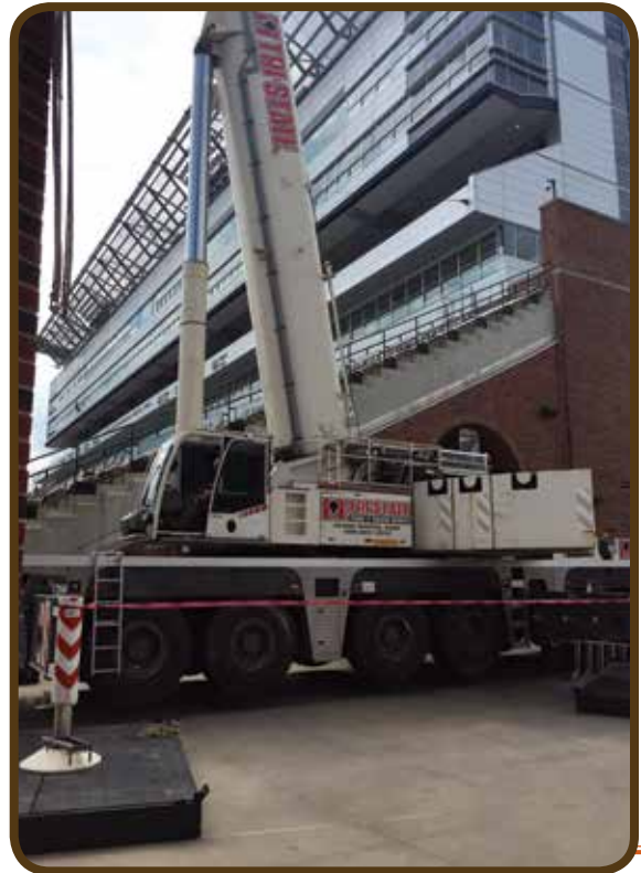
Brother Eric Wincentsen operates a 400 ton crane for Tri-State Crane & Rigging in Iowa City at Kinnick Stadium in preparation for the Back Porch Revival concert
