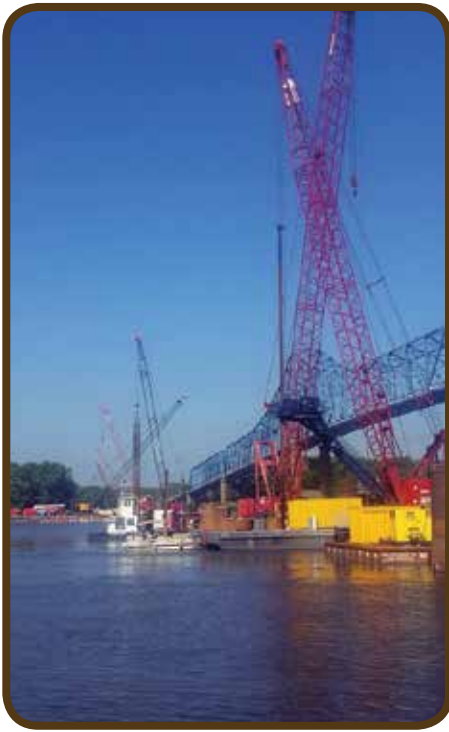
Members of Local 234 and Local 150 working on the Sabula/Savanna bridge project over the Mississippi River
