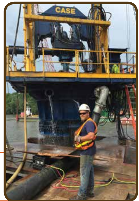
Apprentice Dale Camp working for Case Foundation at the Sabula/Savanna bridge project
