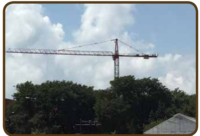
Brother John Connolly operates a tower crane at Bessey Hall on the Iowa State University Campus in Ames
