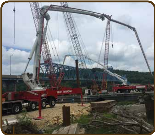
Brothers Matt Drees and Chris Lawrence operate concrete pump trucks for Sun Concrete at the Sabula/Savannah bridge project over the Mississippi River
