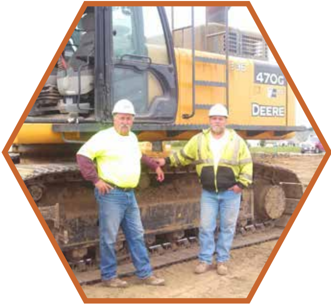
Brothers Dave Acker and Tony Menuey work on a new housing development in Cedar Falls for Dave Schmitt Construction.
