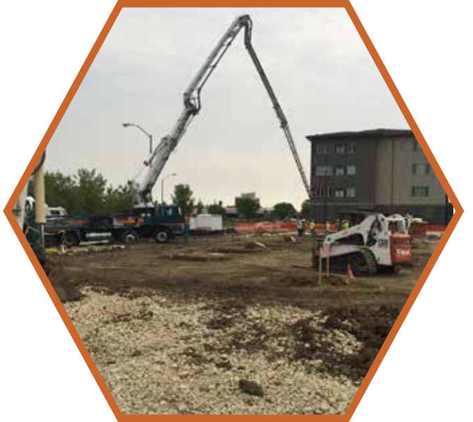
Premier Concrete, pumping concrete on a new condo development in Des Moines.
