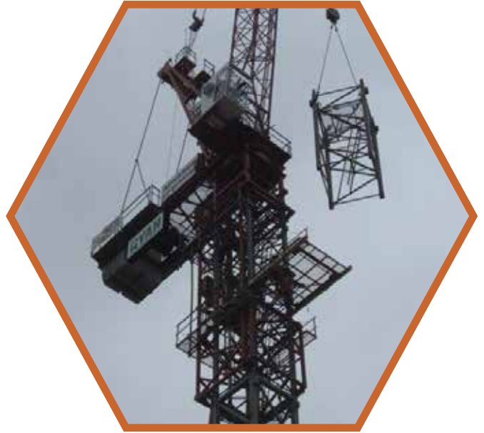
Brother Russ Werner working for Ryan Companies on a new CRST building in downtown Cedar Rapids performing a 70 foot jump with a 160 Wolffkran.
