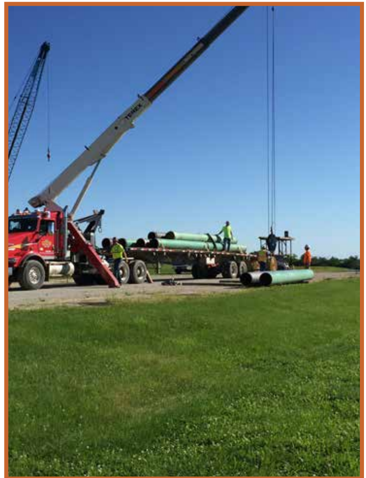
20 inch pipe being off loaded at the training site donated by Precision Pipeline.
