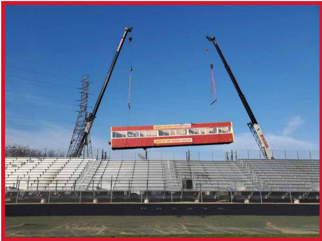
Brothers Nate Lucas and Brennan Rawson operate a 75 ton and a 60 ton crane to take down the Marion High School's damaged pressbox
