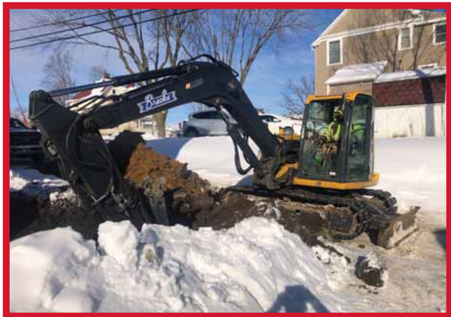
Brother Keith Woods operates a John Deere 85 g excavator for B.G. Brecke digging up a sewer line in Cedar Rapids
