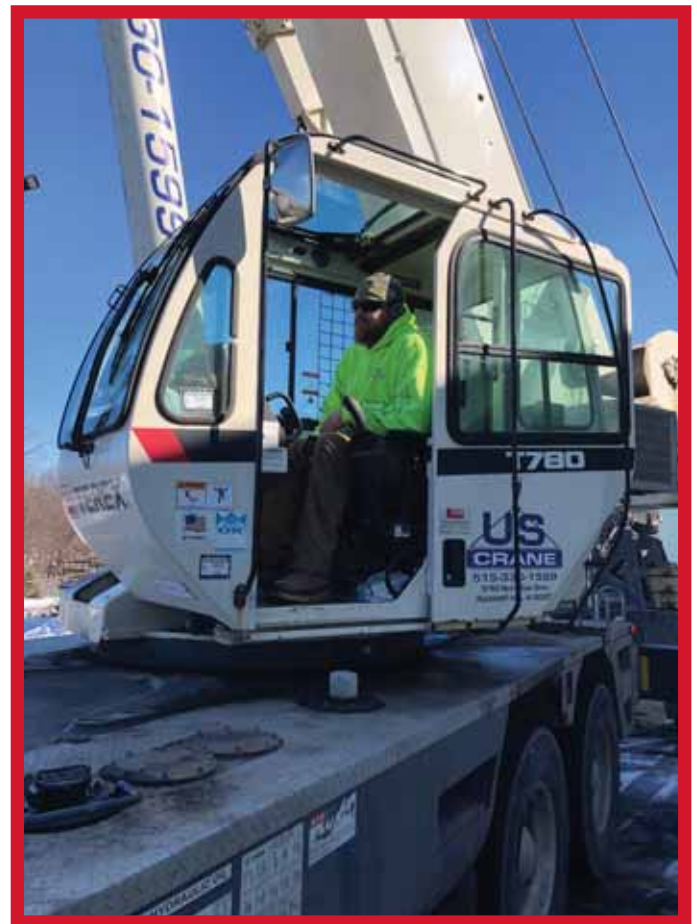
Brother Casey O'Dell operates a T700 setting material for the roofers at the Days Inn on Merle Hay Road in Des Moines
