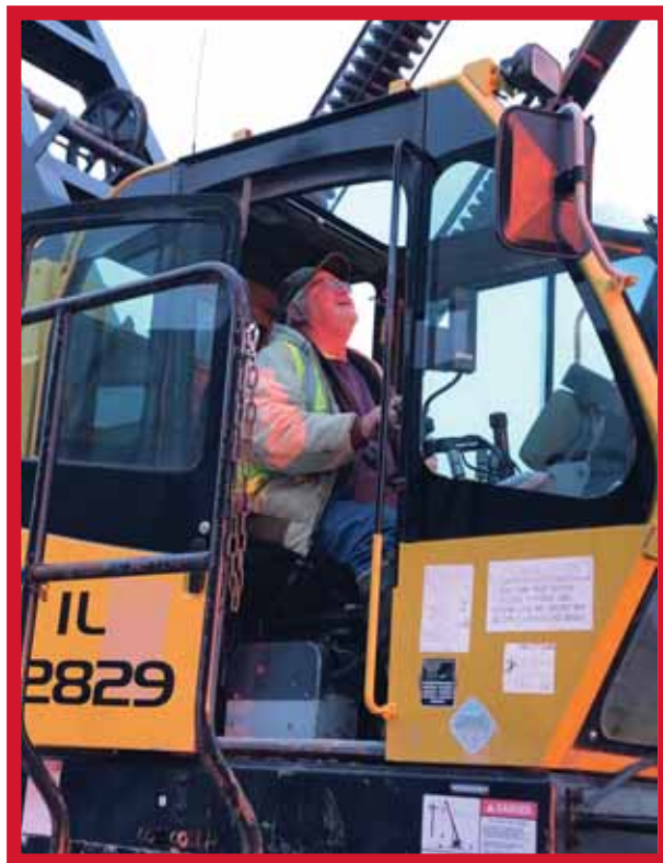
Brother Joel Macken operates a 160 ton Kobelco setting Precast for Northwest Steel Erection at a warehouse in Grimes.
