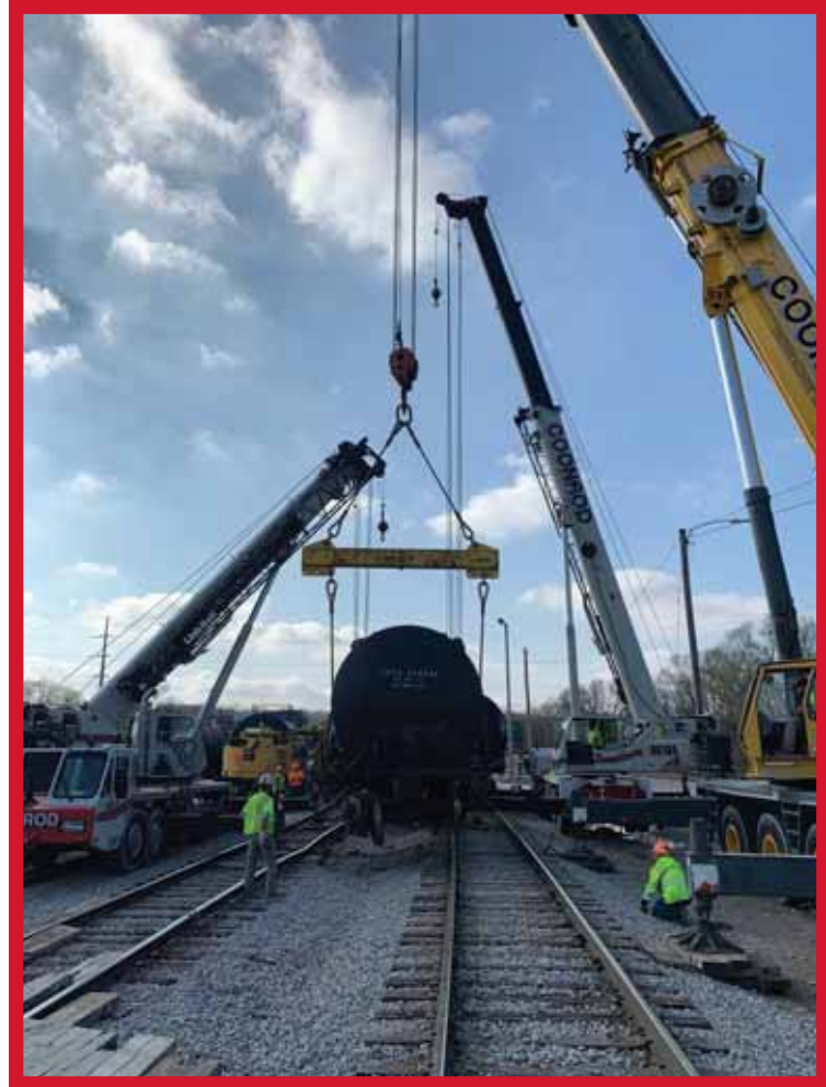
Brothers Tim Carson, Dustin Choplick and Brandon Spicer rerailed a loaded tanker near ADM in Cedar Rapids for Coonrod
