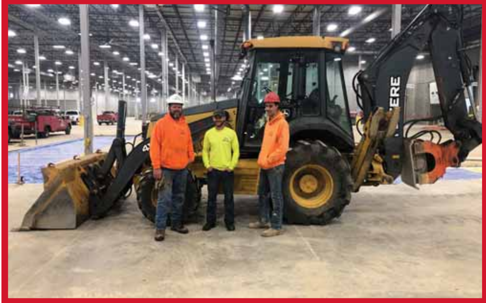
Brother Members JJ Hefel, Tony Jasper and Trevor Gotto working at the new pet food factory for Portzen Construction in Dubuque
