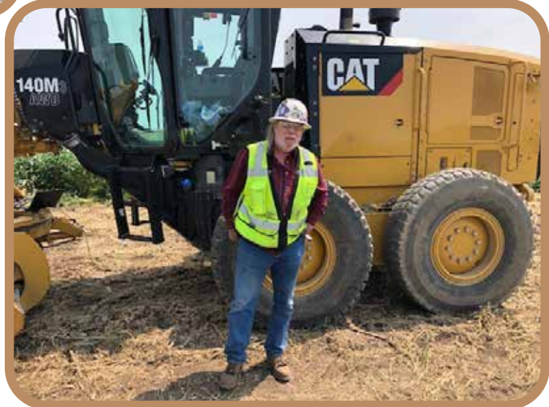
Brother Doug Friend at the new erection project for Mortenson in Sac County
