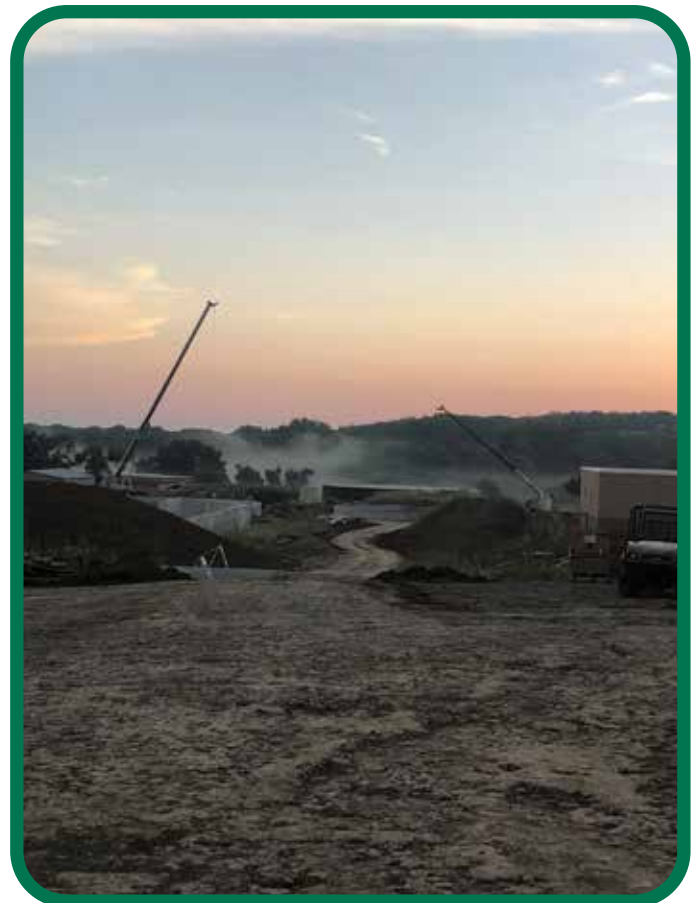
Brothers Kyle Wahlert, Brice Mitchell and Jeremiah Brown at the Indianola Waste Water Treatment Plant for Williams Brothers
