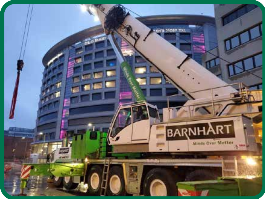
Brother Lee Muldoon operates a Grove GMK 6300L 350 ton for Barnhart at the Iowa City at the University of Iowa Hospital
