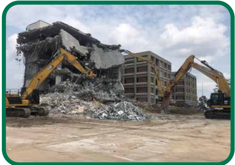
Brothers Brandon Zinser, Brad Bulanda and Michael Whitters demoing the Transamerica building in Cedar Rapids for Zinser Wrecking
