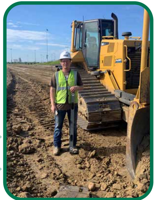
Apprentice Zane Hatfield operates a dozer and checks grade for Elder Corporation
