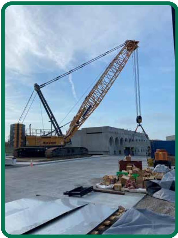
Brother Kyle Jones operates a Liebherr LR 1300 setting storage modules and Brother Chase Schaller, oiler, for Sarens at the Duane Arnold Nuclear Plant in Palo
