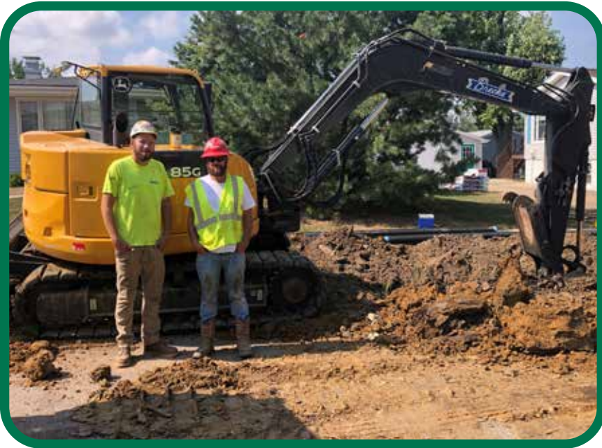
Brothers Ben Brecht and Nick Klein work for B.G. Brecke on a sub drain project in Marion
