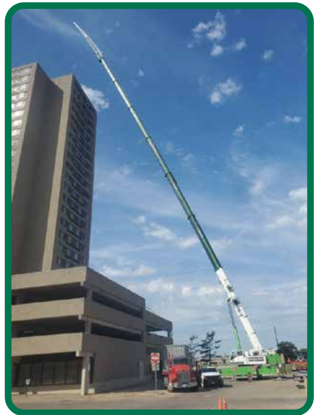
Brother Lee Muldoon operates a Grove GMK 6300L 350 ton for Barnhart at the Iowa Reality Building in Cedar Rapids
