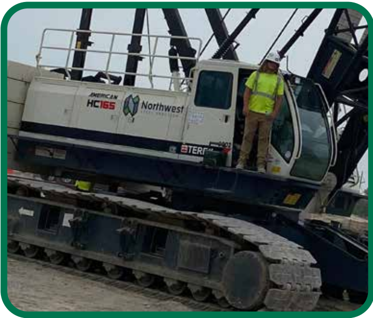
Apprentice Lane Bindel fills in on the 165 ton lattice boom crawler for Northwest
