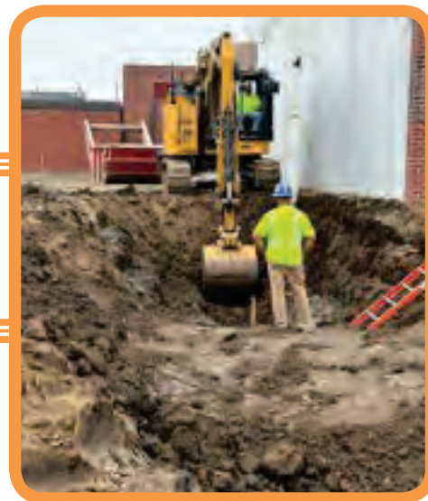
Brother Randy Howard digging pipe for Elder at the Grandview Christian Elementary in Norwoodville
