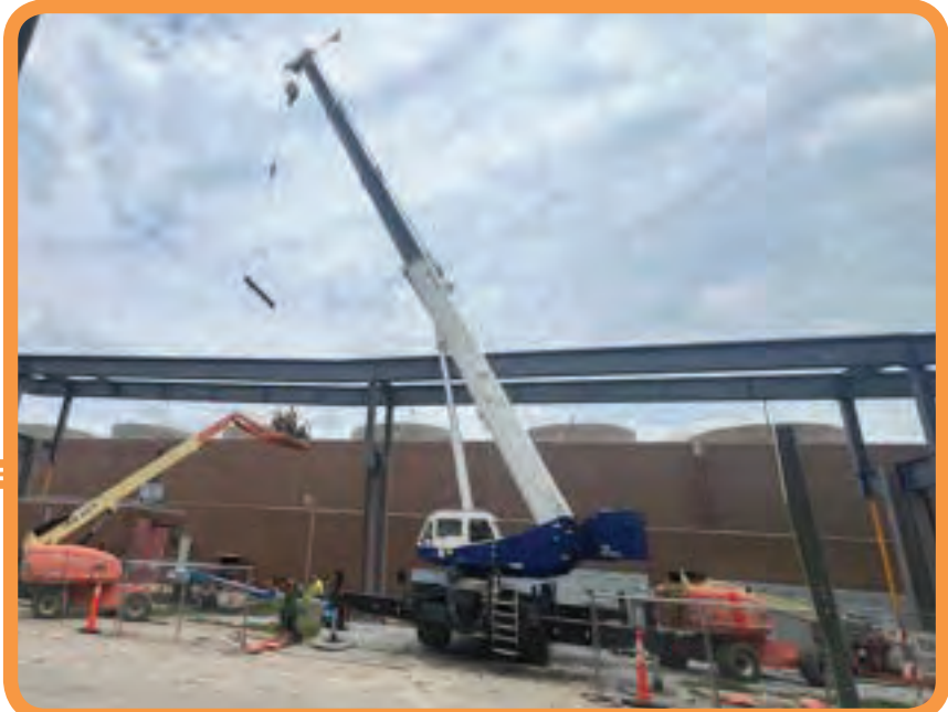
Brother Mitchel Mundorf operates a Tadano GR-900 XL RT crane at the parking ramp skywalk project for Tri State Crane in Iowa City
