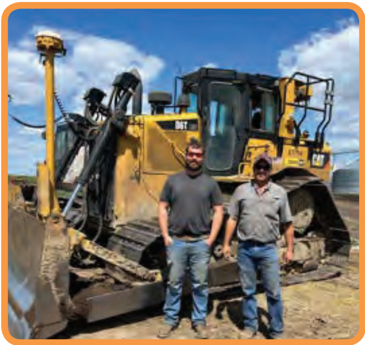
Brother Thad McVey and Apprentice Caden VanHemert working on a housing development in Winterset for Sandstone
