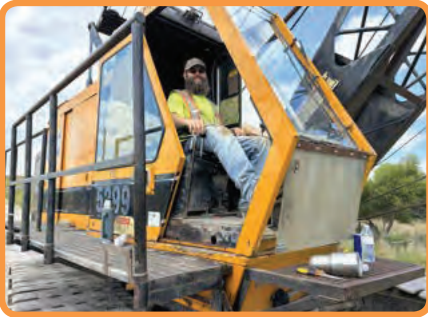
Brother Brad Hill operates an American Friction Rig for Herberger Construction building a bridge in Union County near Creston
