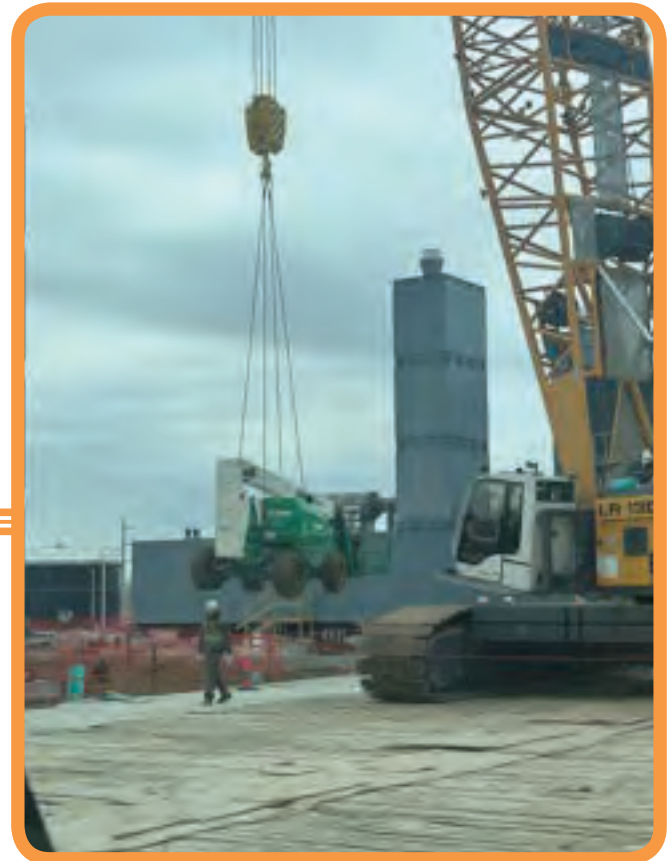
Brother Jordan Buck operates a Liebherr LR 1300 Crawler Crane for JE Dunn at the Council Bluffs Data Center
