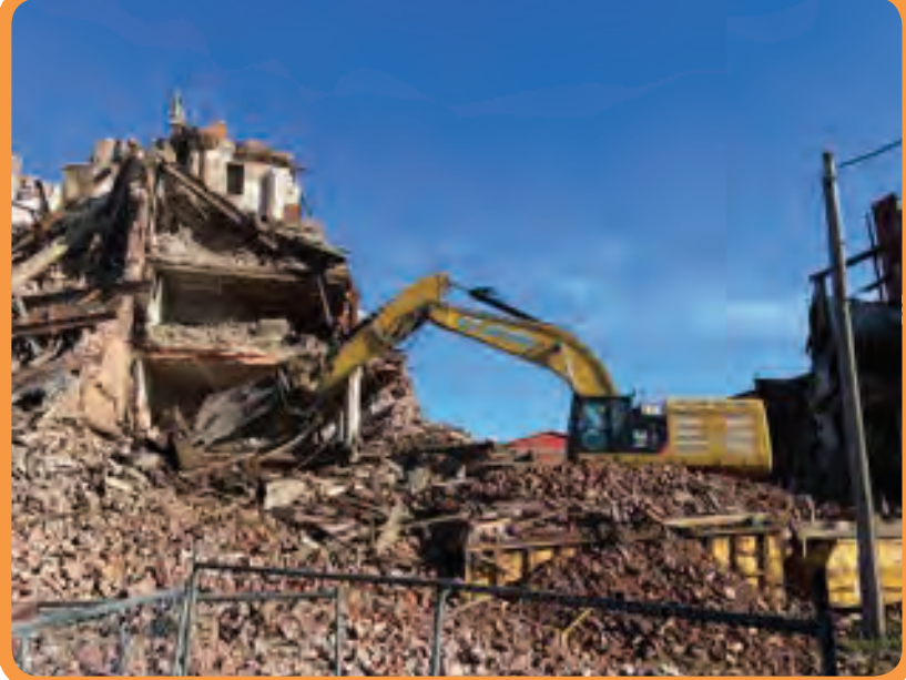
Brother Brad Bulanda is operating a Caterpillar 374 excavator for Zinser at the H&W Building in Dubuque
