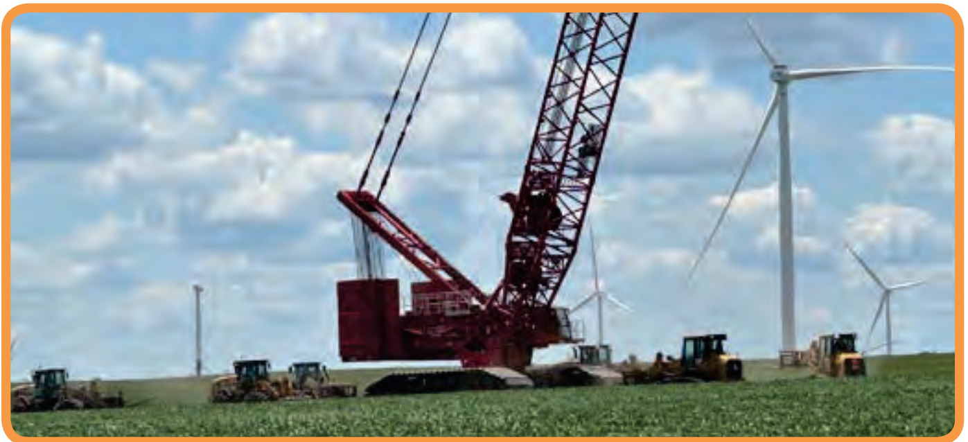
Local 234 operators moving a MCL 650 crane at the Mortenson wind farm repower project in the Tama area
