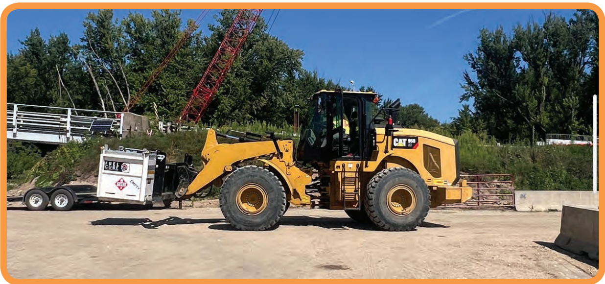
Brother Gary McDermott operates a Caterpillar 950 loader for Kraemer North America at the Lansing Mississippi River Bridge project
