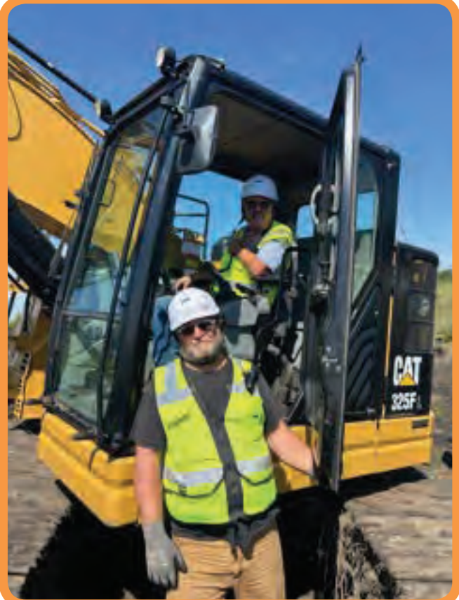
Brother Ken Richardson and Brother Dan Law working for Mortenson at a wind turbine project near Emmetsburg
