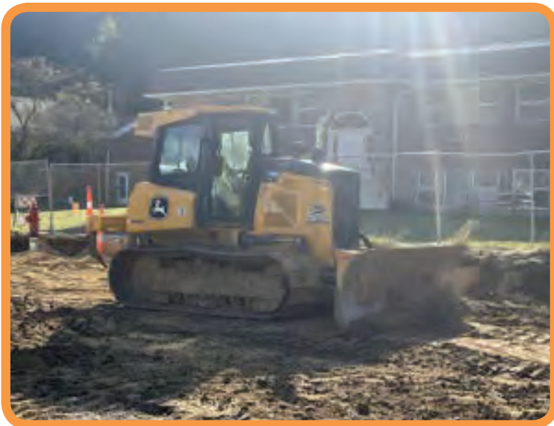
Apprentice Alan Hohensee working for Portzen on a street project in McGregor
