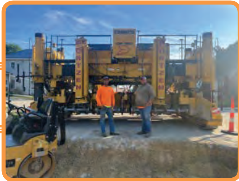
Brother Mitch Schueller and Brother Jeremy Langel working for Portzen Construction on a street project in McGregor
